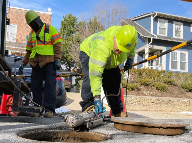
Jeff Harden, a closed-circuit television operator conducts an inspection of sanitary sewer lines.
