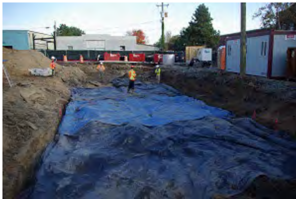
Above Left: It is important to keep the site covered to help protect the wooden features of this building and keep them wet until the archaeologists are ready to remove them.
